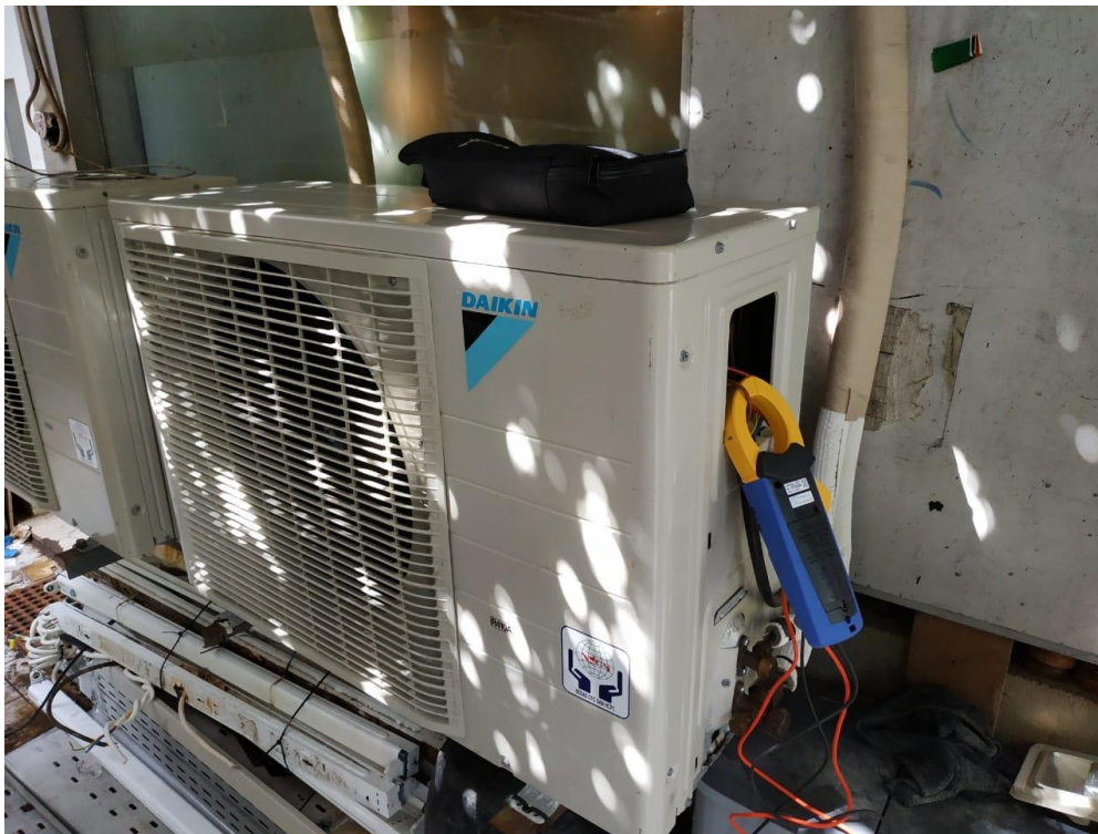
FIGURE 1. POWER LOGGING USING HIOKI CLAMP ON POWER TESTER ON A AC COMPRESSOR AT PHBC.
